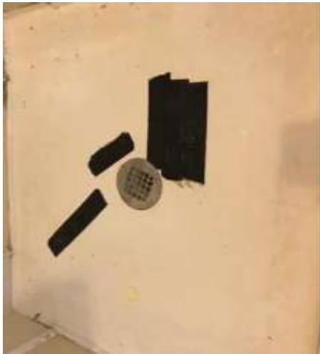
Cracked Shower Stall Floor
