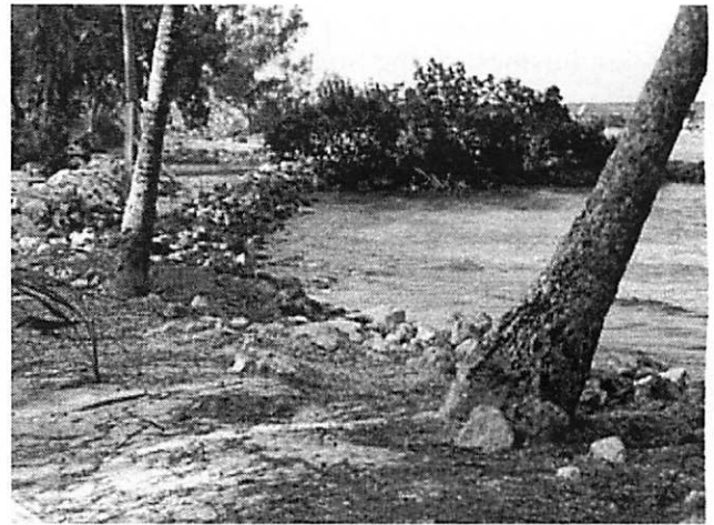
Figure 4. Erosion south of old groyne fronting cabins. This groyne is longer than the others and has been effective in trapping sand.
