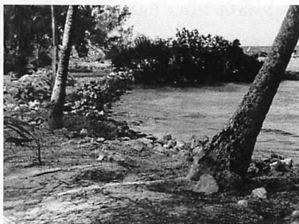
Figure 4. Erosion behind small groyne (in background).
