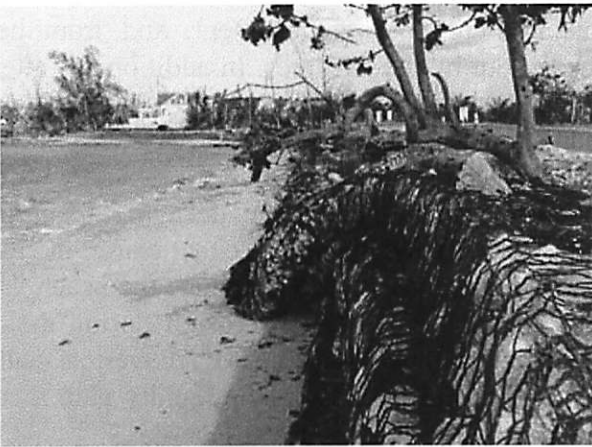
Figure 5. Collapsed gabion along West bay Street, Nassau, 2002.
